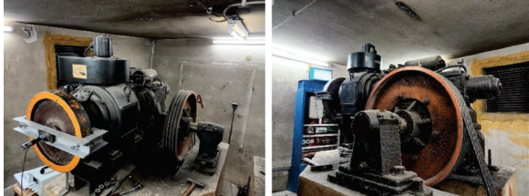
Fig. 8. Driving machine of passenger elevator
